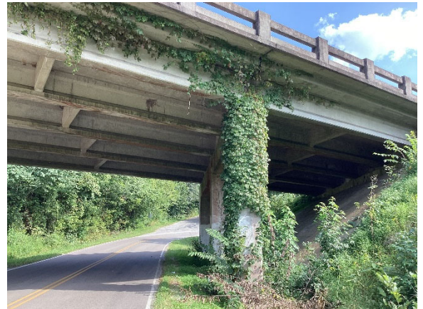
Figure 19 – Overgrown vegetation underneath I-65 bridge in Giles County
