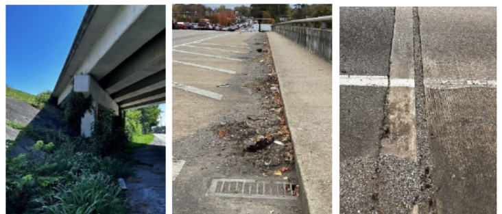
Figure 21 - Common bridge issues: overgrown vegetation, clogged scupper pan from lack of sweeping, joints filled with dirt and silt
